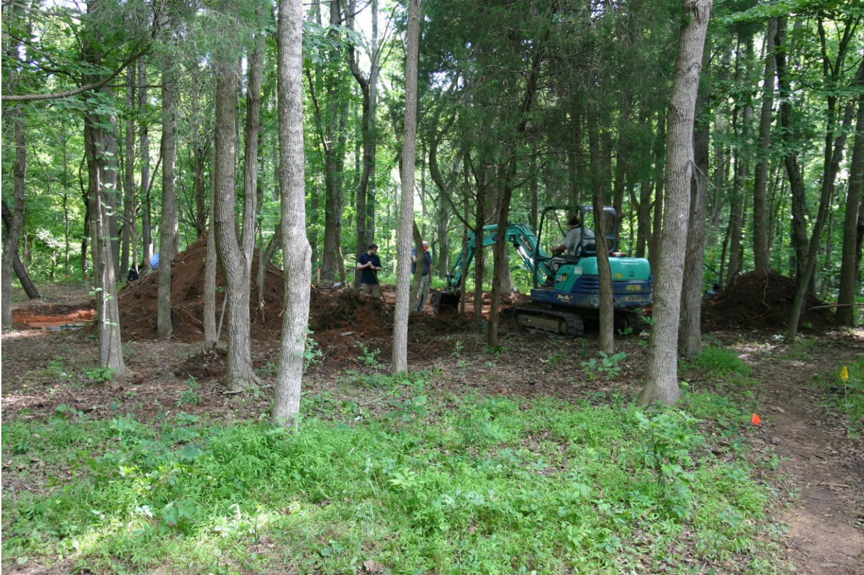
Figure 3.12. Stripping topsoil from Ayers Town with a mini-excavator during the summer 2010 field season. View to southeast.
