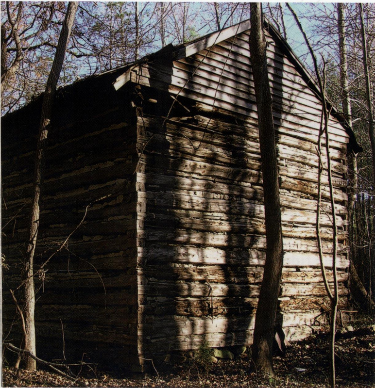
Most old tobacco barns such as this one on the Duke Forest have collapsed and their foundations are all that remain. Duke Forest Photo Collection.
